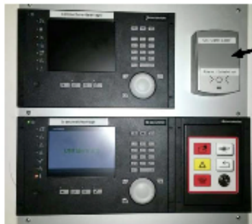
Card reader for resetting the burglar alarm with the UniCard
